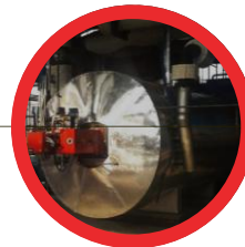
3.5 MW Thermal Oil Heater for Biscuit Baking
